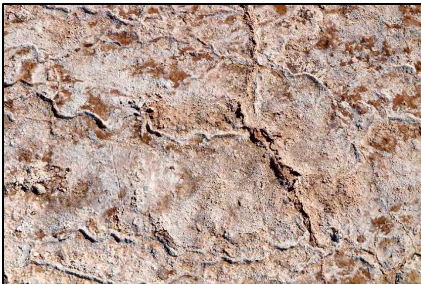
Figure S10-8. White crust in drainage. X-ray diffraction identified halite and thenardite in the material. Photo by W. Hood.
